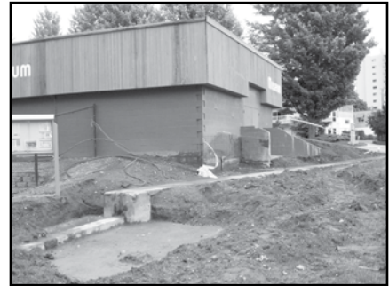
City workers removed a tree and dirt to expose the 1940s dike. In the foreground is where the railroad track came through. Workers filled it with concrete, Sept. 2013.
